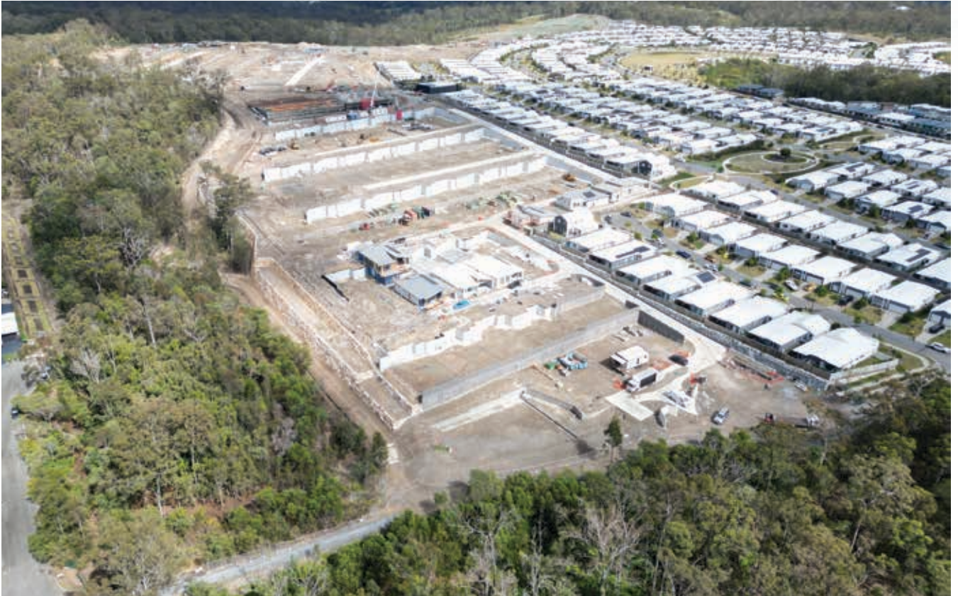
STAGE TWO RESIDENTIAL CONSTRUCTION COMMENCED IN Q3 2023 AND STAGE ONE RESIDENTS MOVED INTO THEIR BRAND NEW HOMES IN Q4 2023
