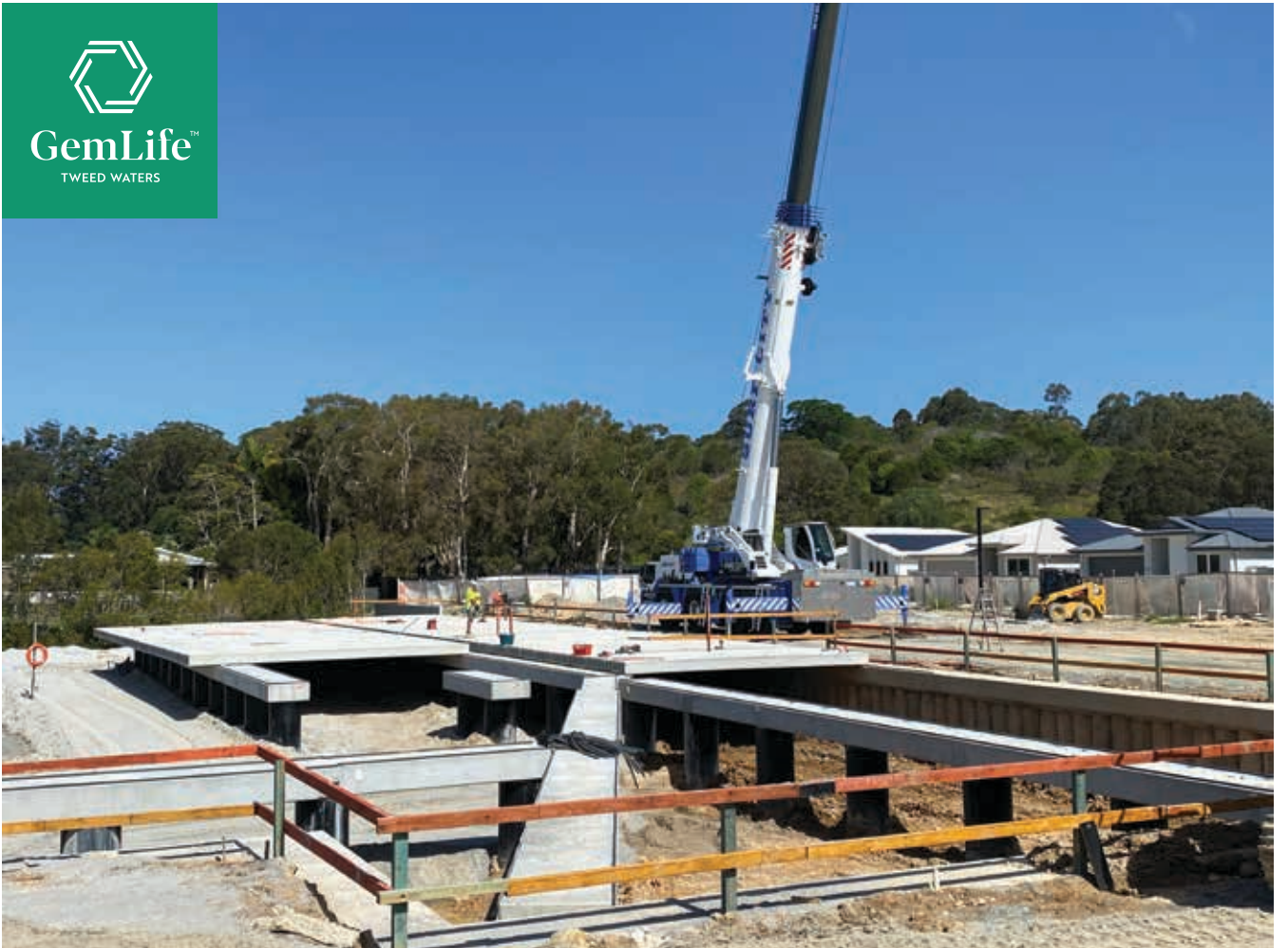
FIRST HOMEOWNERS MOVED IN IN Q4 2023 AND WORK IS PROGRESSING WELL ON THE WATERFRONT COUNTRY CLUB, WITH THE GROUND SLAB COMPLETED
