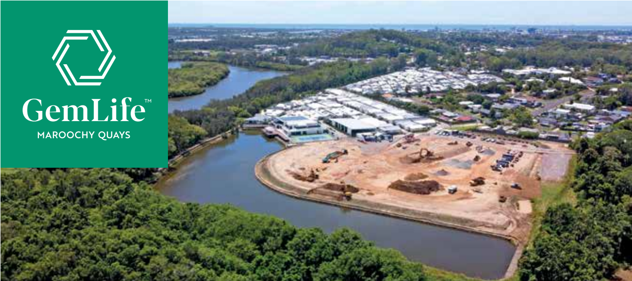
CONSTRUCTION FOR AN OFF-SITE CARAVAN STORAGE COMPOUND IN KULUIN AND STAGE FOUR OF THE RESORT COMMENCED IN Q3 AND Q4 2022 RESPECTIVELY
